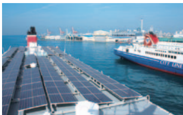
Solar power generation system
